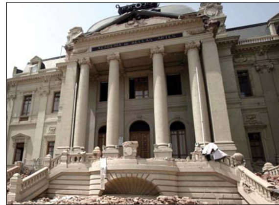
Academy of Fine Arts building in Santiago after a huge 8.8 magnitude earthquake rocked Chile on February 27, 2010
